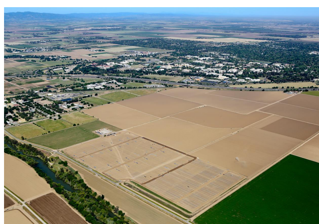
The beginning phases of installation of 62 Acre Sun Power solar farm on the south eastern portion of UC Davis campus. Photo taken 2015, courtesy UC Davis Utilities.
